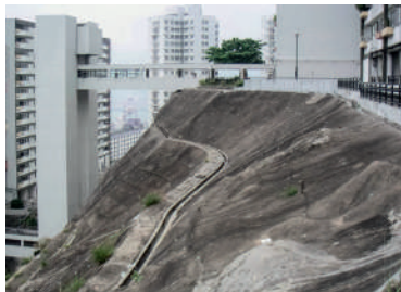
13 The entire slope is covered with a concrete skin to prevent landslides due to the loose soil consistency of the hill. This protection includes controlling and drainage systems as well as a network of pathways and stairs.
