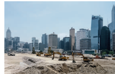
15 Land reclamation 2008, Hong Kong Island-Star Ferry Pier area: while Land reclamation was stopped in Victoria Harbour due to environmental issues, it is still an important factor for the government to generate revenues by leasing the newly constructed land.
