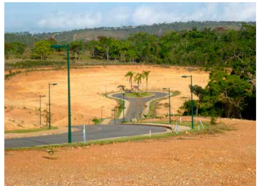
Land clearance for the construction of “Reserva Real,” north of Lagoa Santa
